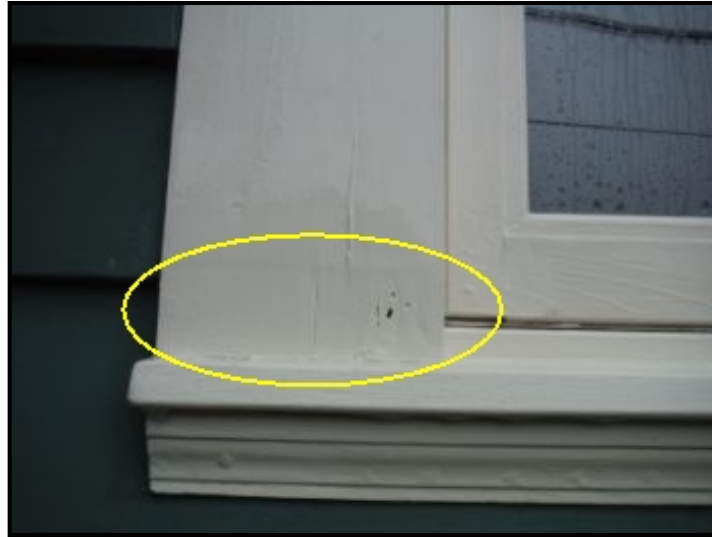
Small area of soft wood at south side window trim.
