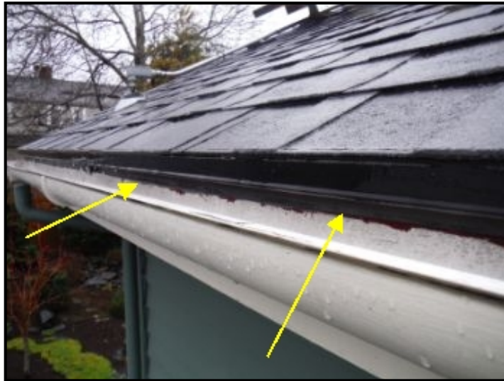
Sample of gutter drip edge flashing being too short.
