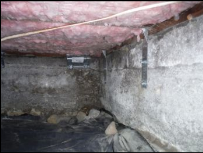
Partial view of the crawlspace under the living room. Note the seismic bracing.
