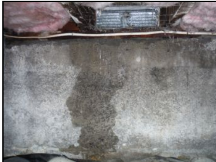
Evidence of moisture intrusion through vent screen.
