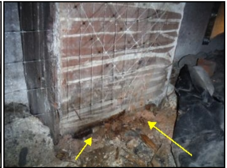
Wood / soil contact with rot present.
