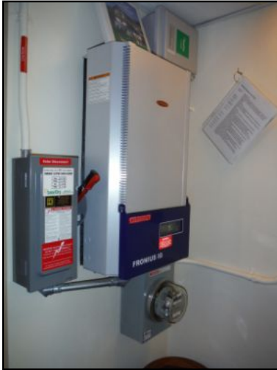
This is panel and controls for the solar power.
