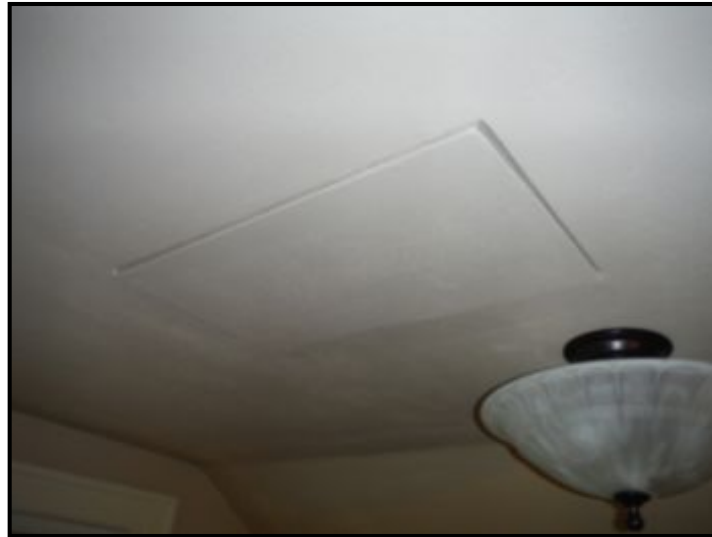
View of the minimally sized attic access.
