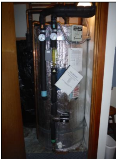
View of the insulation wrapped water heater.
