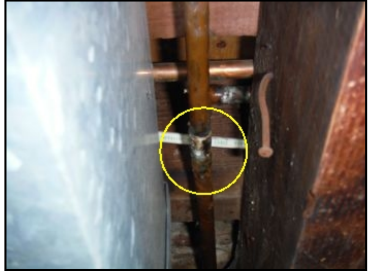
There is small leak at in the furnace room.
