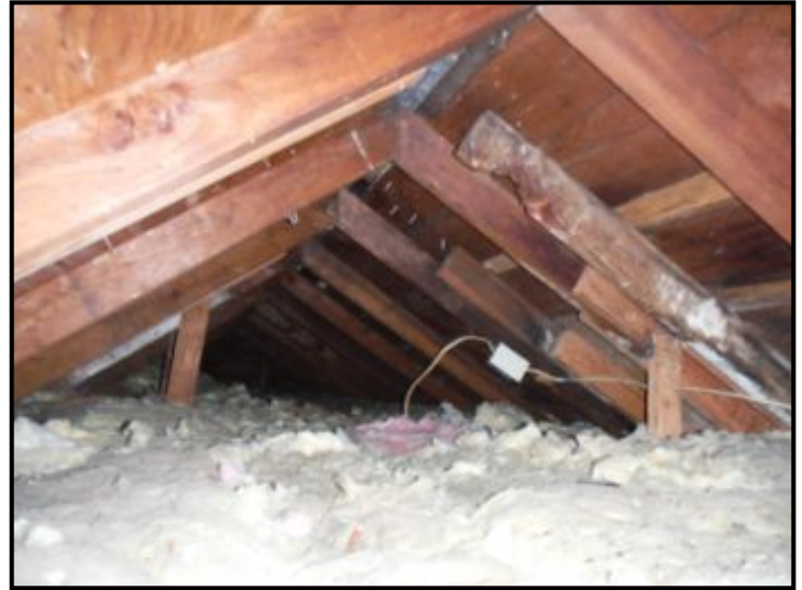
Evidence of framing alterations in the upper attic.
