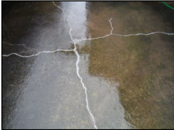
Sample of cracking in the driveway concrete.
