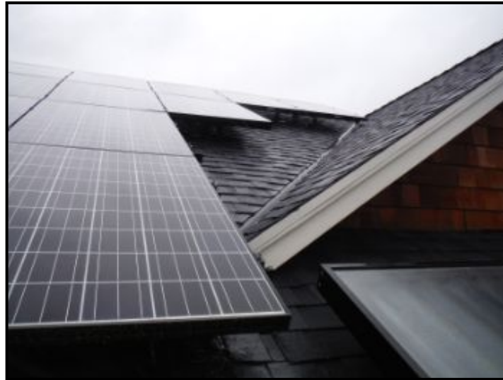
Partial view of the roof and installed solar panels.
