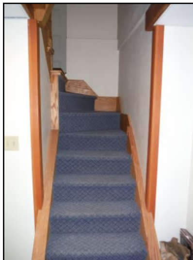
The width, riser height and lack of handrail would not meet today's building standards.
