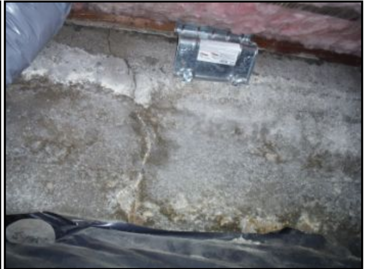
Sample of a foundation crack.
